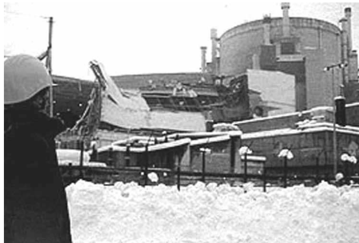
Figure 2.5 Superphénix collapsed turbine hall roof. Photo: Dissident-Media.
