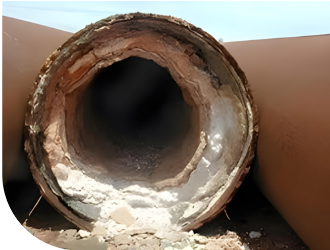
Figure 3 - Oil Pipe with NORM Scale
